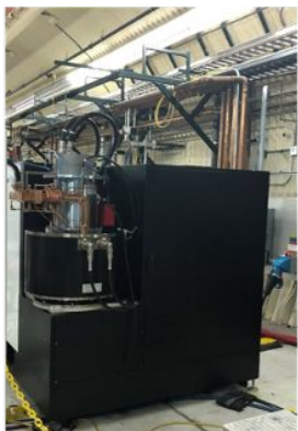
New 50 MW peak power C-band klystron installed in September 2019
