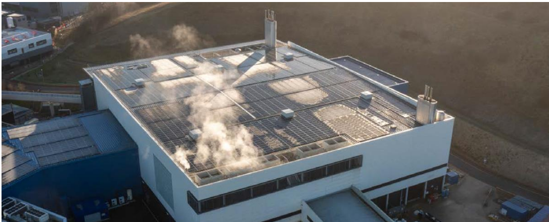
The old coolers in action
