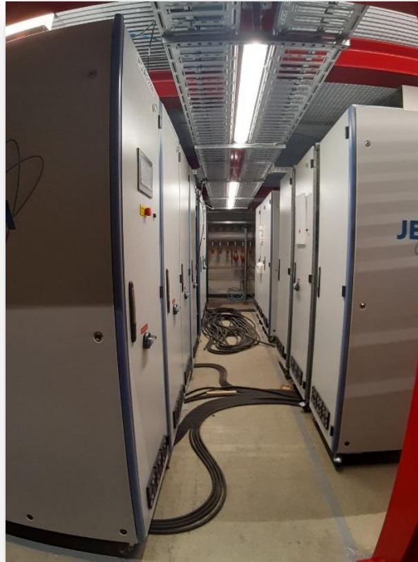
17 modules of 20-kW 1300-MHz solid state amplifiers
