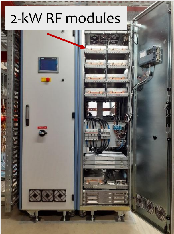
20-kW 1300-MHz control unit and power supply
