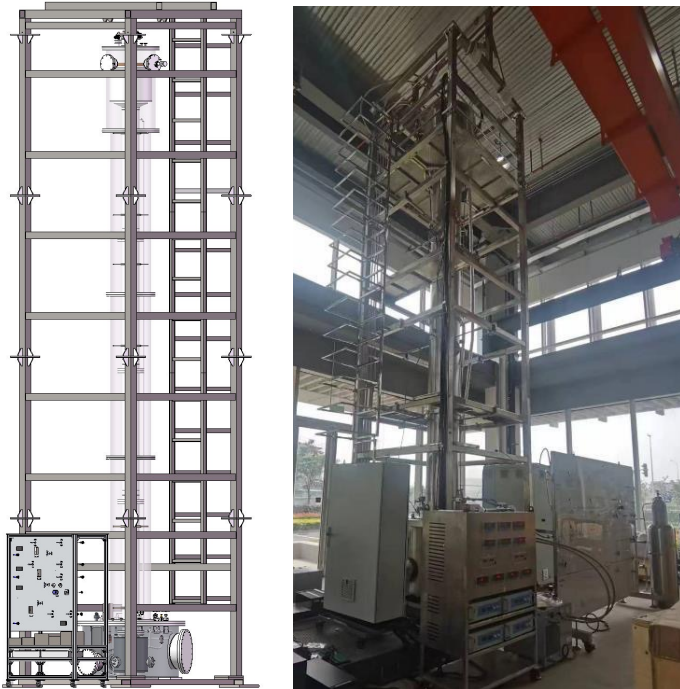
Krypton distillation tower
