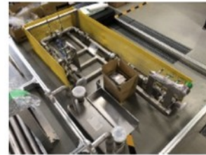
New target cooling system
