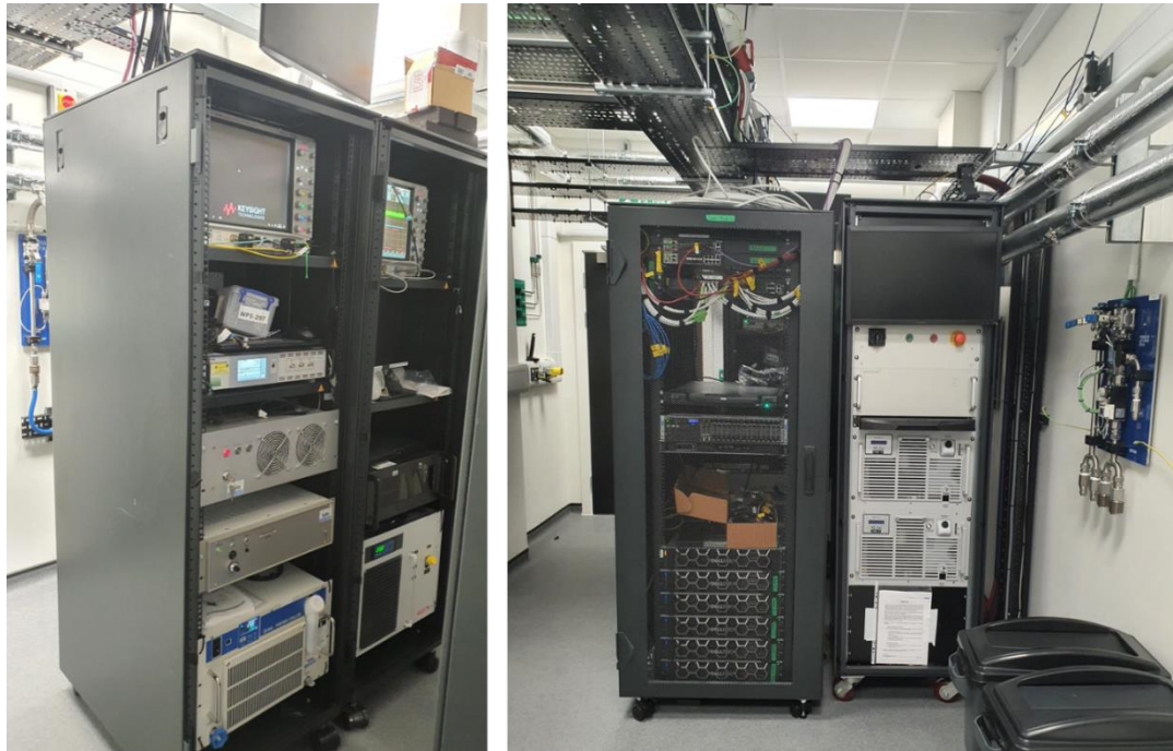
Figure 28: Rack room racks, displaying the Front-End chillers and the timing system (left) and the 10 J cooling system (right)
